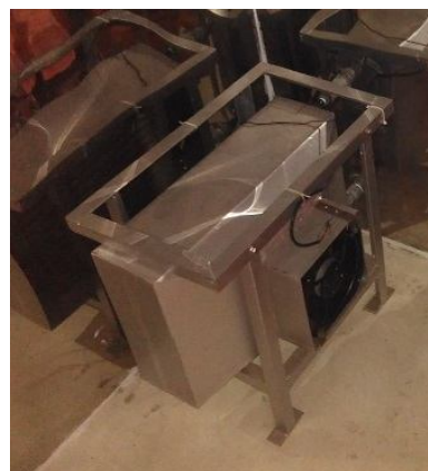
Fig. 5. Hot water fed to air heat exchanger
