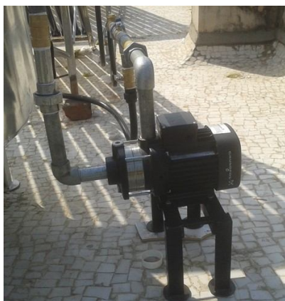
Fig. 4. Pump for hot water circulation
